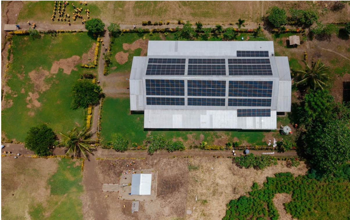
Installation of solar panels at the Sir Dudley Tuti College Chapel as part of the Solar Hybrid Power System.
